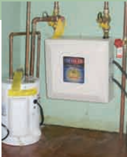
Two backup water heaters, one on-demand and one tankless, provide supplemental water heating for each residence.
