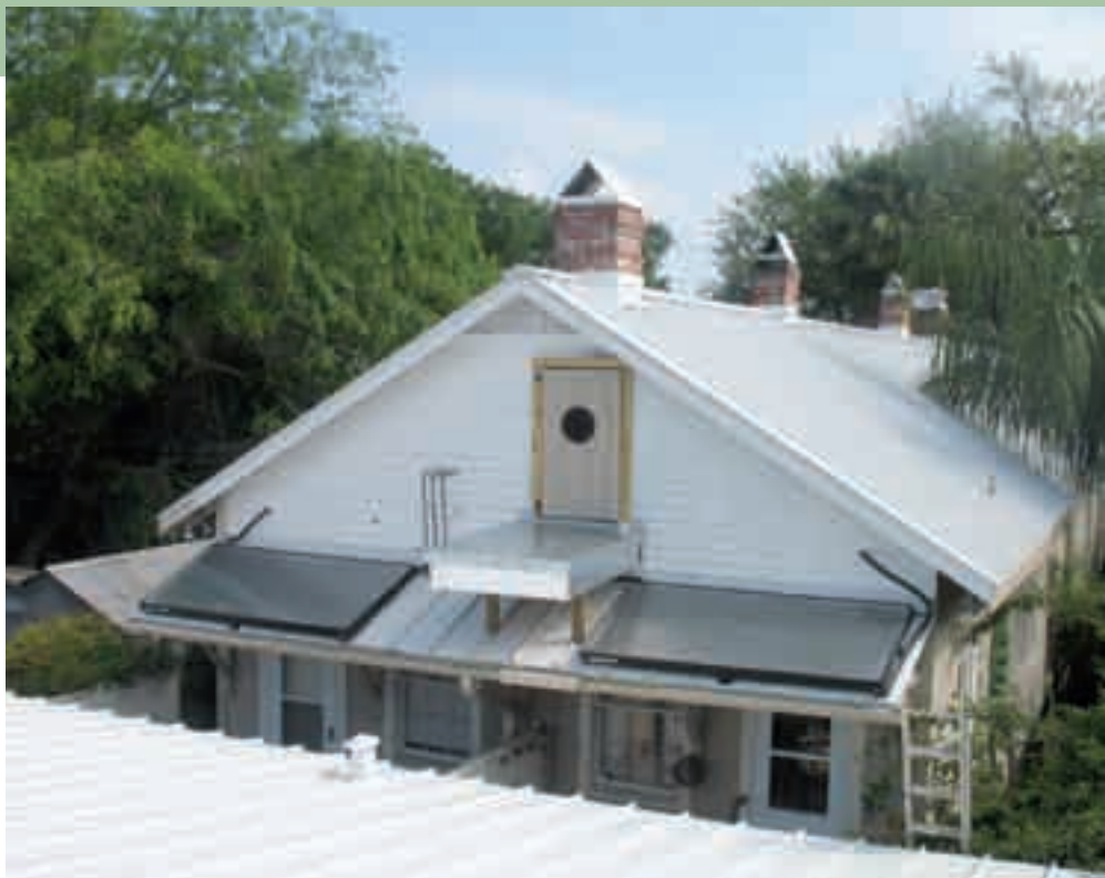
The back porch roof had just enough room for two solar collectors. The staging balcony was left in place to make future system maintenance easier.
