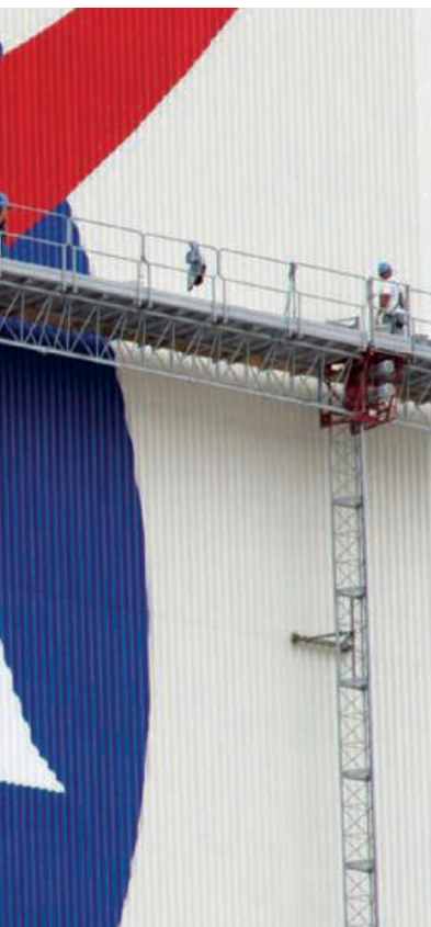
Needs more than a lick of paint
