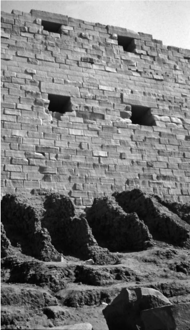
Fig. 5.7. The remains of a mud-brick construction ramp against the inner face of the first pylon of the Temple of Amun at Karnak.
